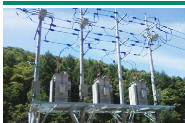
Picture of Installation Case (PVR 7,000kVA)
