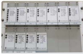
TD Panel (Station)
