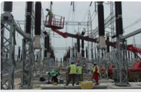
CT & PT Commissioning Test (330kV SWYD)
