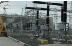
C.B Commissioning Test (330kV SWYD)
