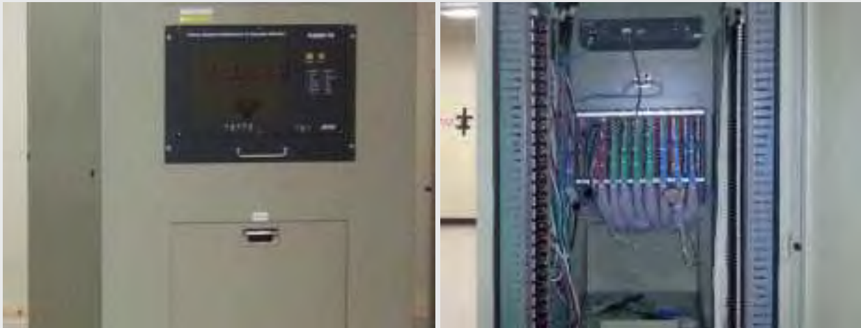
Fault recorder installed in Hanul Plant 1 (Front/Back)
