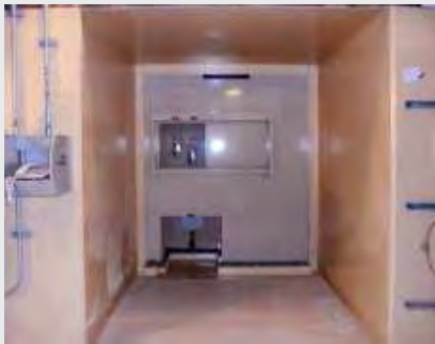
Post-Accident Sample Sink (Front)
