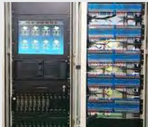
System cabinet (Kori unit 1)
