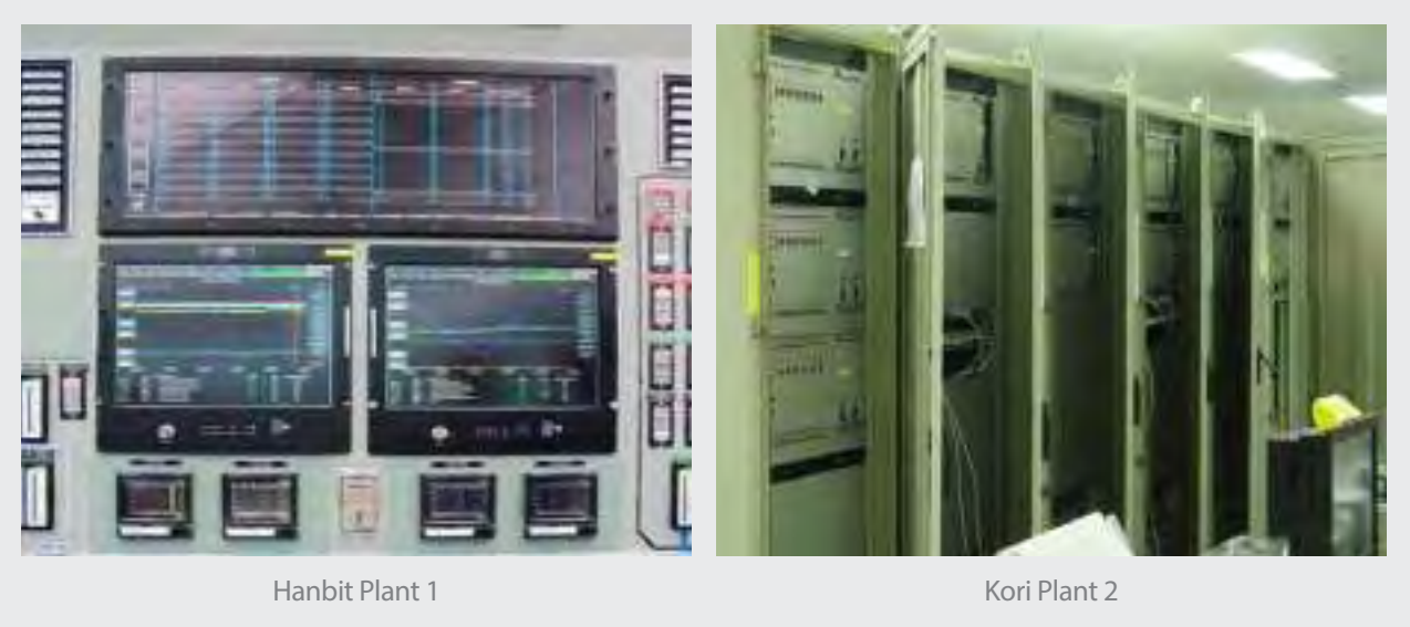
[Plant Monitoring System]
