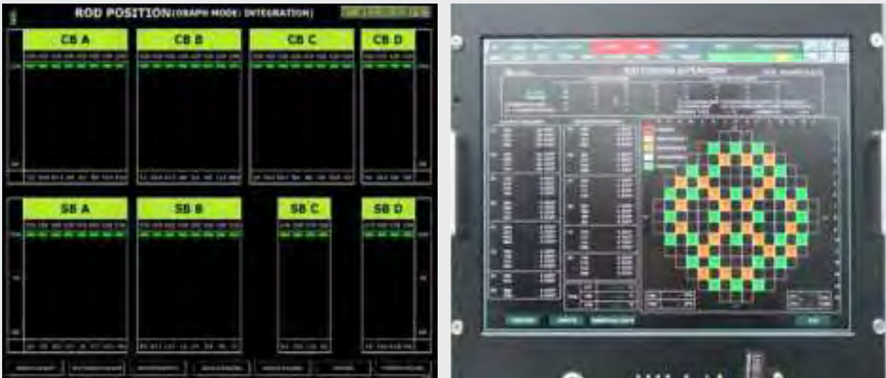
User Interface Screen (Kori Unit 3 Main Control Room)
