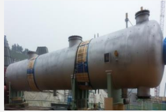
L.P. Feed Water Heater
