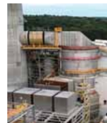
Experience : PSNH Merrimack Power Station, Unit 1 & 2 Location : Bow, New Hampshire, USA Customer : PSNH Start-Up Year : 2012 Capacity : 457 MWe Flue Gas Flow : 1,688,000 Nm 3 /h
