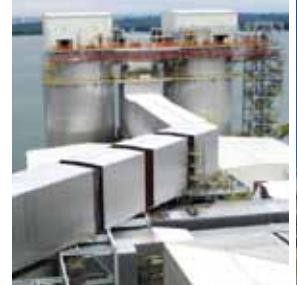
Spray Dryer Absorber (SDA) Largest SDA Reference : 3 x 600 MW
