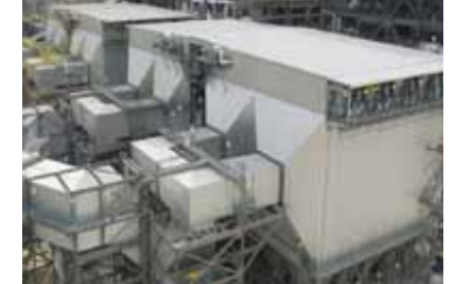
Particulate Control Dry Electrostatic Precipitator (DESP) Design : 4 x HaRDE ESP Capacity : 2 x 600 MW
