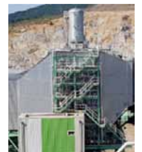
Non-Leakage GGH Reheater Design : 1 x Horizontal Flow Spiral Fin-Tube with Enamel Coating
