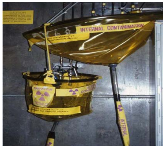
FIG. 8. Drip bags used for leaks (when allowed by regulator). (Courtesy of Pacific Gas & Electric Company, USA).
