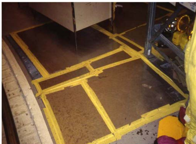
FIG. 35. Reusable metal plate over floor grating. (Courtesy of Pacific Gas & Electric Company, USA).
