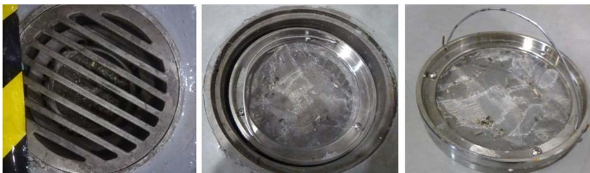
FIG. 9. Installing a metal filter on floor drain to remove solids. (Courtesy of Pacific Gas & Electric Company, USA).
