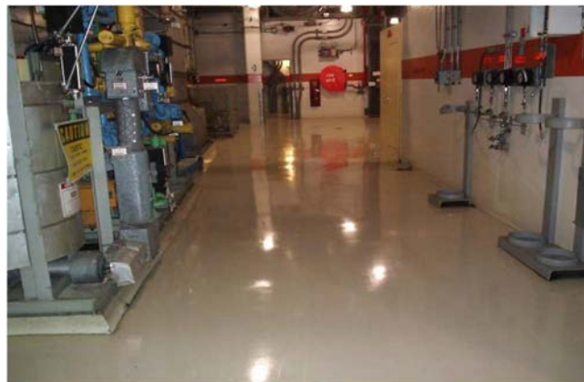
FIG. 28. Floor coatings replacing disposable plastic sheets. (Courtesy of Pacific Gas & Electric Company, USA).
