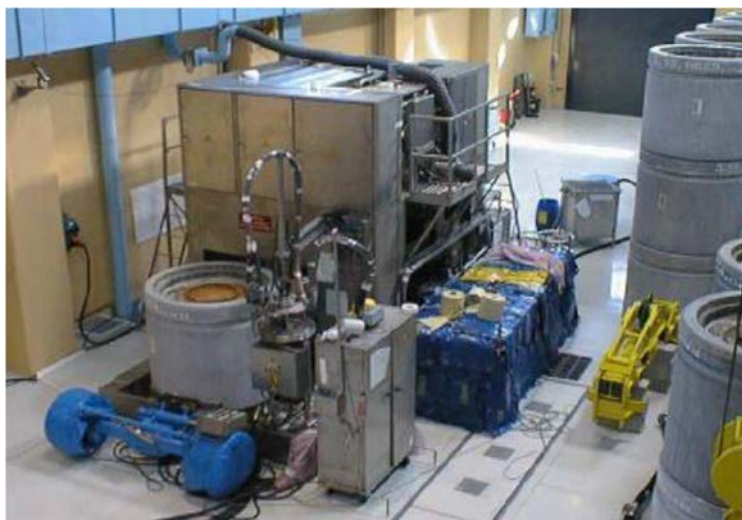
FIG. II-2. MERCURE Process in operation at production site. (Courtesy of EDF, France).
