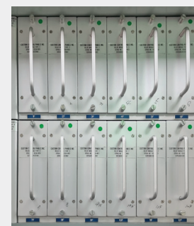
Heavy Water Reactor Type(CANDU / 700MW)SDS#1 PDC-RELAY MODULE
