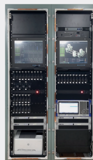
NIMS(INSSS Integrity Monitoring System) Cabinet
